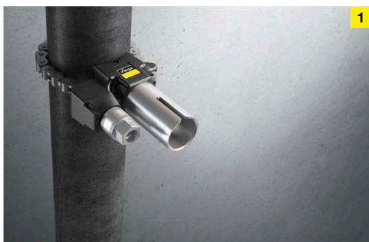
1. Attach a special drill guide on the steel pipe to guide the drilling shaft.
